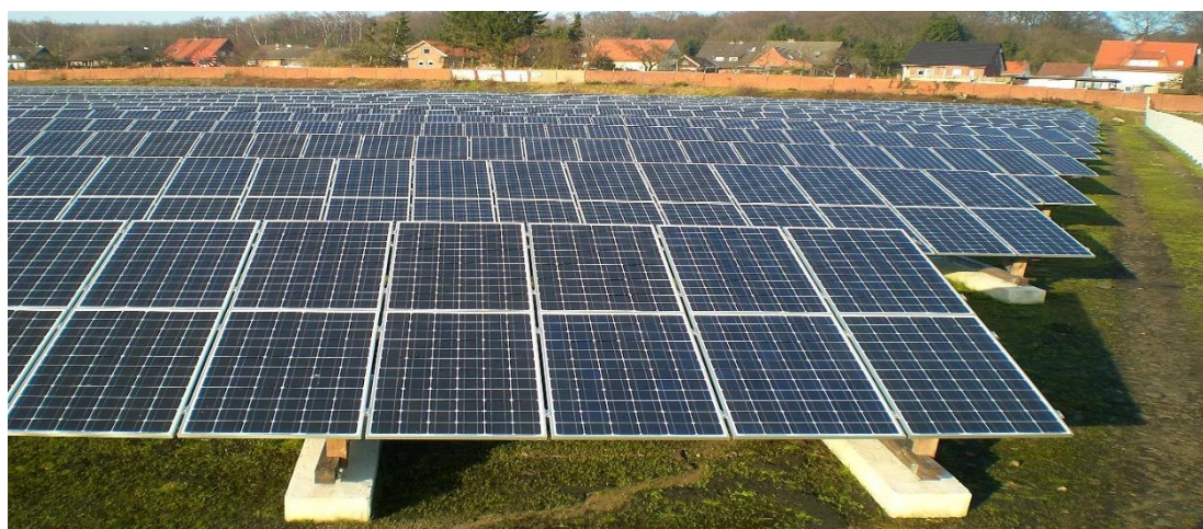
Figure 7 Ground mount PV system (Mohamed Amer Chaaban, 2017)
