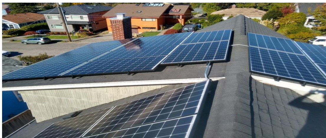
Figure 69 Roof mount residential system (Sayre, 2020)
