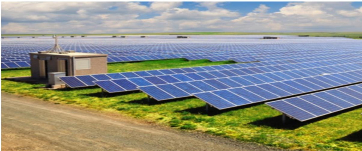
Figure 46 The ground installed system (VE, 2020)
