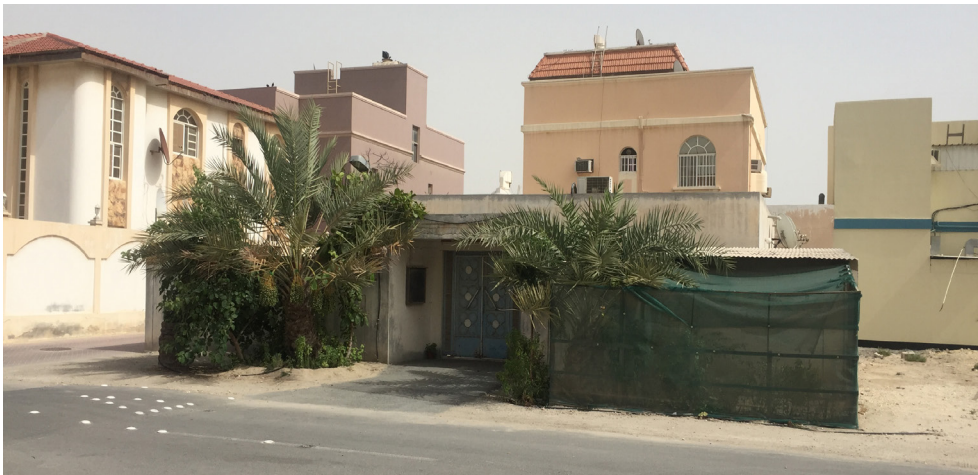
Figure 3: The house which needed refurbishment and students participated in its refurbishment proposal (Islam Abohela 2017).
