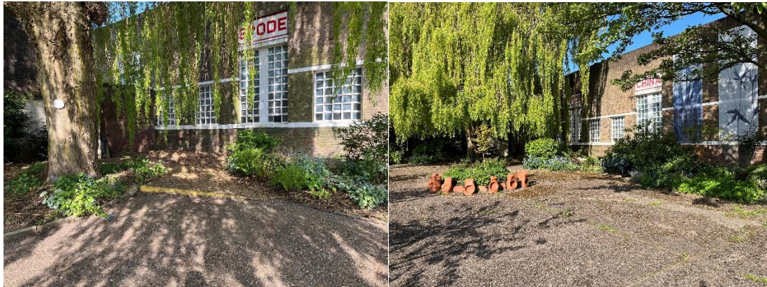
End section of the garden, where we would extend the planting and create flint and reclaimed kiln furniture paths, as hard standing would not work here due to the willow tree's roots which are currently pushing up the concrete. And image of the cracked pavement.
